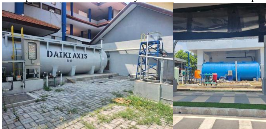
Figure 17. Wastewater Treatment Plant (WWTP) in UNAIR Source: Directorate of Logistics, Security, Order, and Environment, 2024
